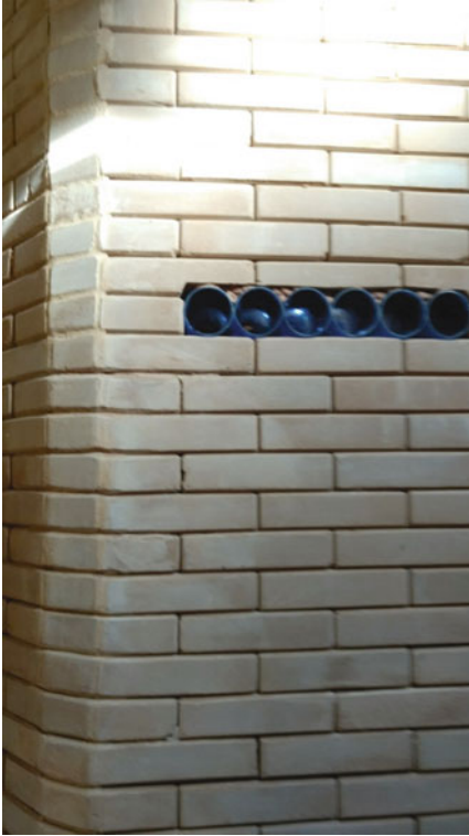
Bio-construction Potential for Sustainability in São Paulo, Brazil, Fig. 3 Wall made with soil-cement bricks. (Source: The authors 2017)
